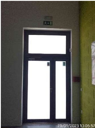
Fire exit and emergency lighting
